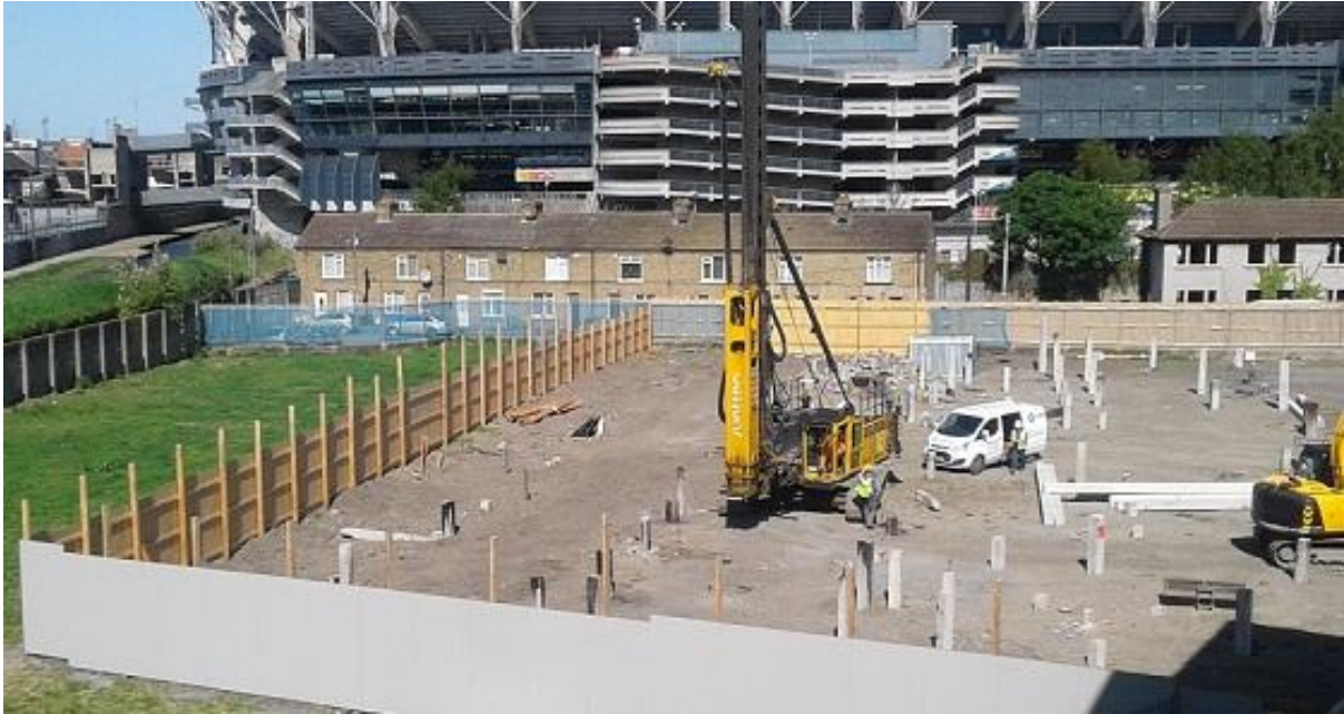
Demolition work on the main construction site at Croke Villas has been completed and construction work is set to begin.
